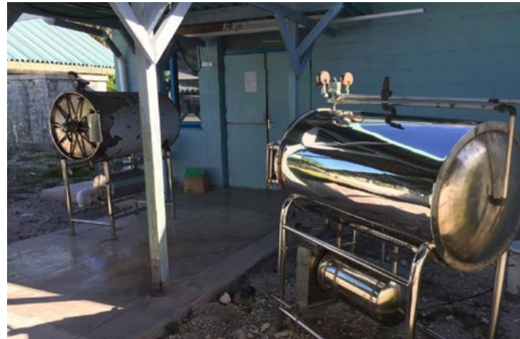
Steam autoclaves no longer in use.
